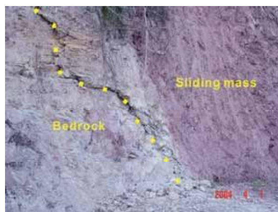
Figure 4 Deformation situation at the right boundary of Block-I outcropped at a roadside
